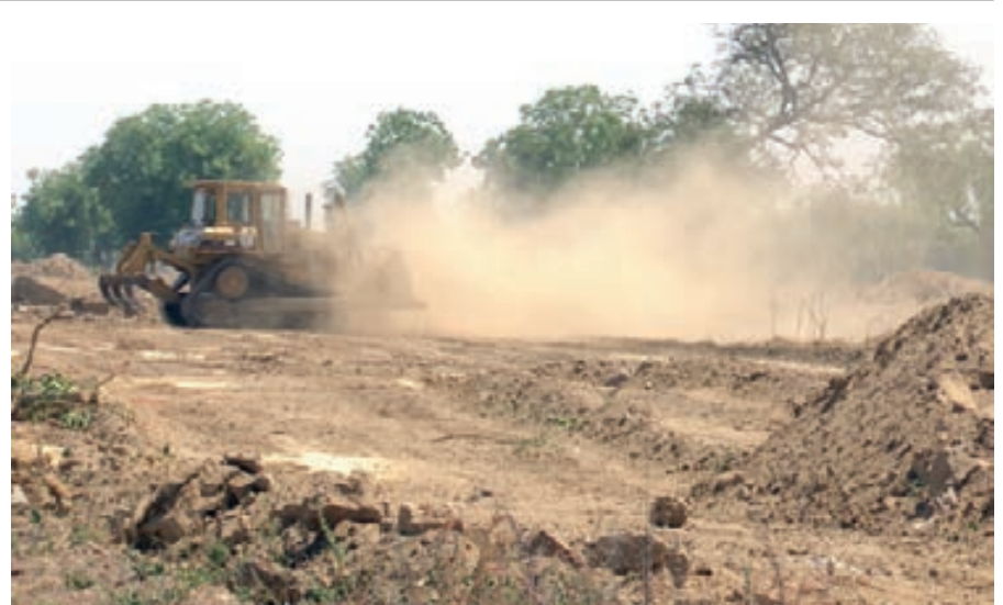
Staff of Kaduna State Urban Development Authority (KASUPDA), using bulldozers to demolish the parameter fence at a land said to belong to the Ahmadu Bello University (ABU), Zaria situated at the College of Agriculture and Animal Science, Mando in Igabi LGA of Kaduna State, yesterday
