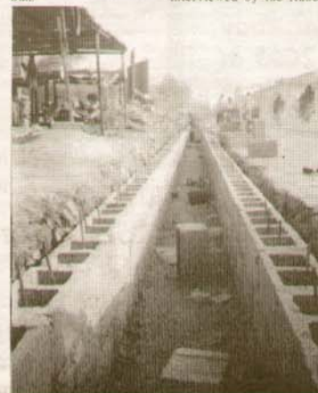
Construction of drainage along Yan by Sarkin Jaki Road, by Governor Shekarau administration.
