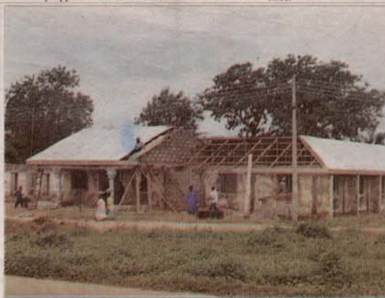
Renovation work on the Gwagwalada LEA secretariat now completed by the Gwagwalada area council administration.
