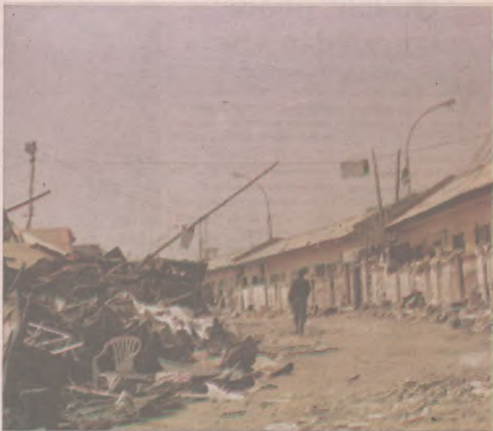
Demolished containers-shops heaped on a major street of the old Wuse Market
