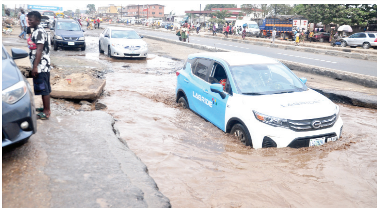
Motorists waded through a dilapidated portion of Lagos-Abeokuta Expressway at Ile-Epo Market in Lagos State
