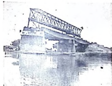
The Hinna Bridge, which spans the Gongola River in North East state, under construction.
