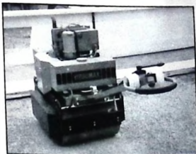
The electrostatic insulators can be seen on the handle assembly
