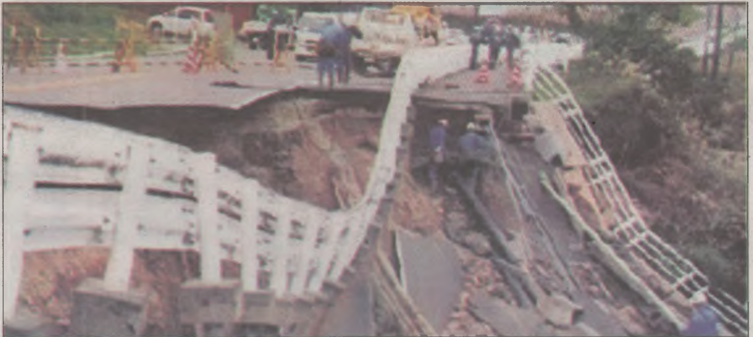
THE earthquake caused widespread destruction including the collapse of major roads
