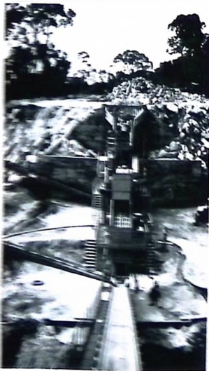
The primary section of a 200 TPH stationary plant in The Ivory Coast
