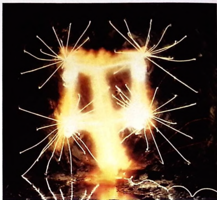
A tunnel round with Nonel - the non-electric blast initiation system that is completely safe to all sorts of electric disturbance, at the same time as the hook-up offers maximum simplicity.
