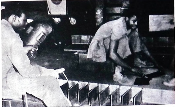
Geilinger is one of Switzerland's oldest manufacturing and contracting firms in the construction sector. Recently it assumed management responsibilities in a Nigerian steel group manufacturing semi-trailers and small steel structures, along with a 30 per cent shareholding. Pictured here, a worker at one of the plants Geilinger is managing.
