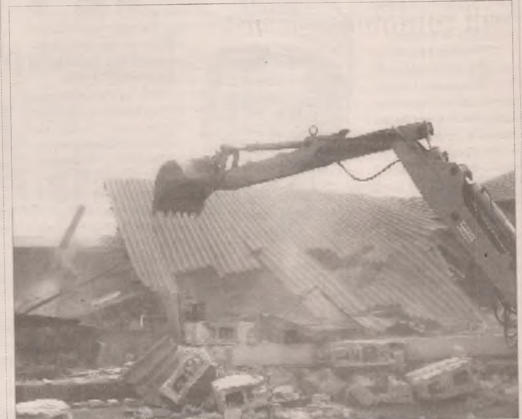
Lagos State urban and regional planning board, demolition squad pulling down shops and containers at the toll gate end of the Lagos-Ibadan expressway...recently
