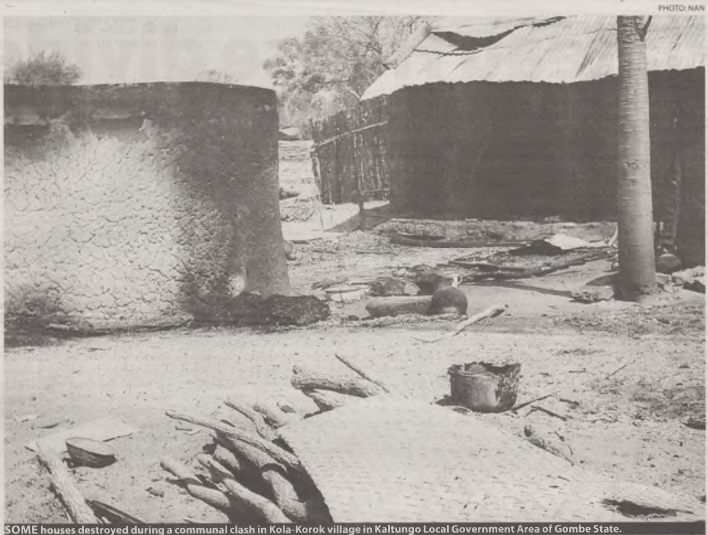
SOME houses destroyed during a communal clash in Kola-Korok village in Kaltungo Local Government Area of Gombe State.
