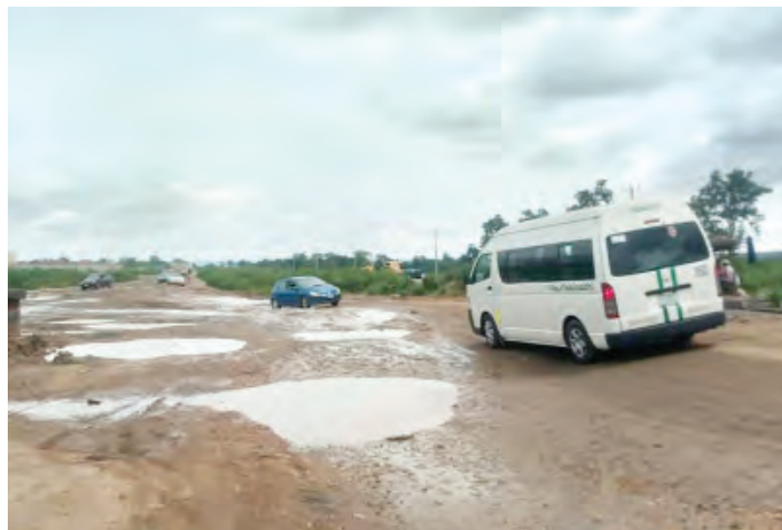
■ A bad section of the road
