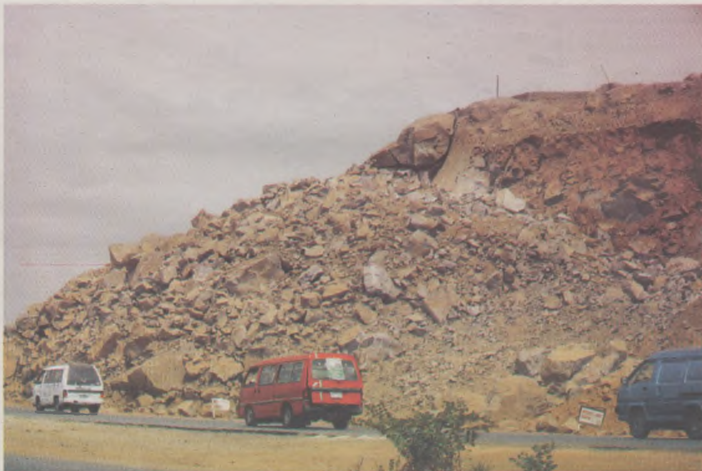
ONGOING drilling of rock to pave way for the dualization of the Kubwa expressway, Abuja
